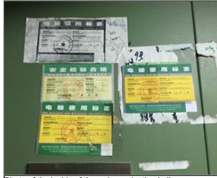
Photo of the inside of the main production hall Elevator-2.JPG
