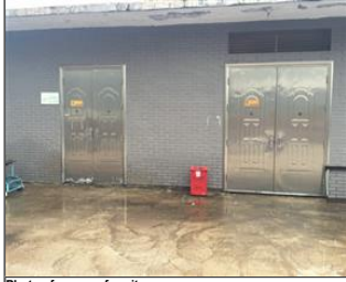
Photo of non-conformity Transformer room without warning labels.JPG
