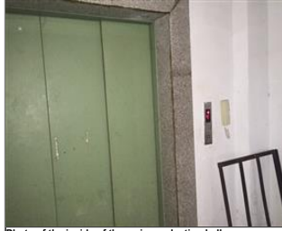
Photo of the inside of the main production hall Elevator-1.JPG
