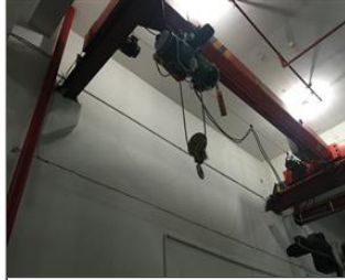
Photo of the inside of the main production hall crane.JPG
