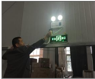
Photo of the inside of the main production hall Emergency light test.JPG
