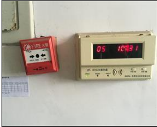
Photo of fire safety equipment fire alarm-2.JPG
