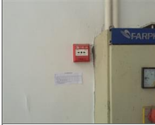
Photo of fire safety equipment fire alarm-1.JPG
