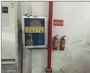
Photo of fire safety equipment fire hydrant.JPG
