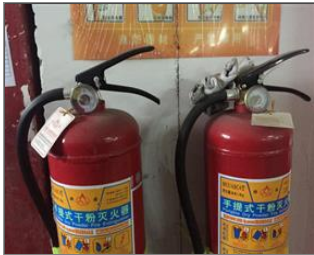
Photo of fire safety equipment Fire extinguisher.JPG
